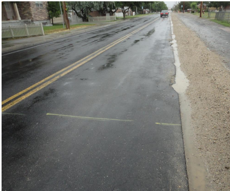
Photo 4. Poor Surface Drainage- (West Valley City)
