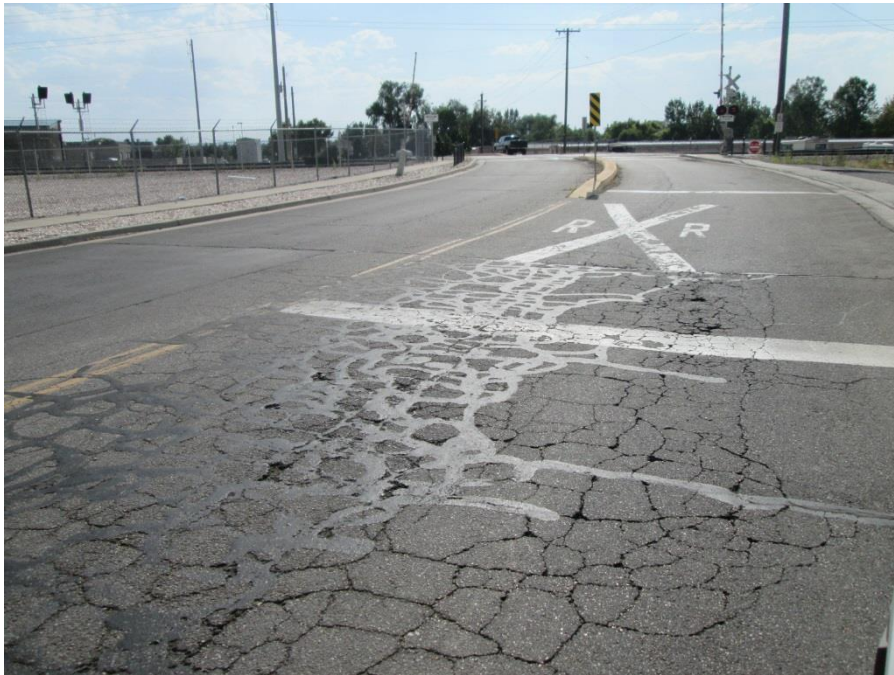
Photo 5. Poor Condition – Old Mill Rd from 600 West to Desert Dr. (RSL = 2 years)
