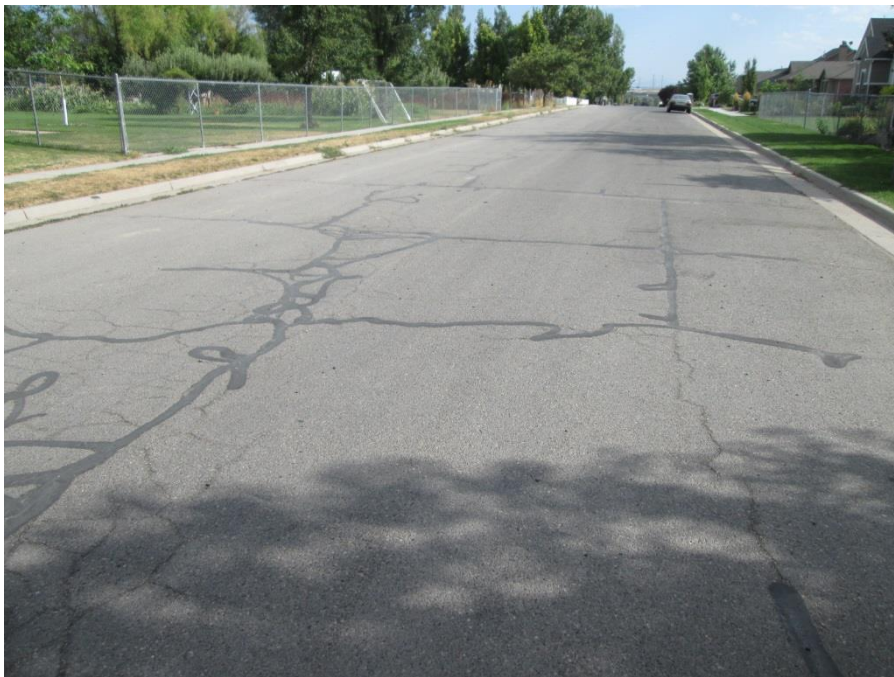
Photo 6. Fair Condition – 50 East from Shepard Ln to 2200 South (RSL = 8 years)
